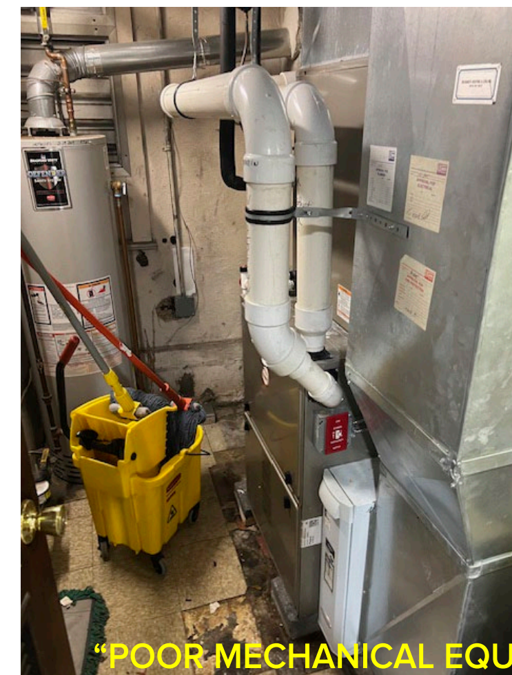
"INADEQUATE WORK AREAS"
